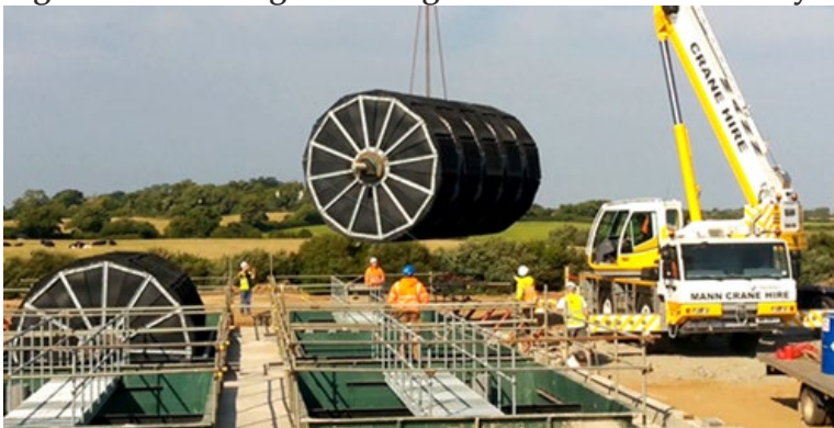
Figure A2.2: Fitting one of eight IRBC rotors at Ramsay's Treatment Works
