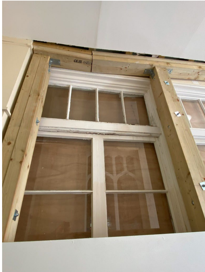
Turner Building – timber framed single glazed windows to the link corridor (either side of the Main Hall): water damage noted to the frames and timber panelling below with the South elevation worse than the North.
