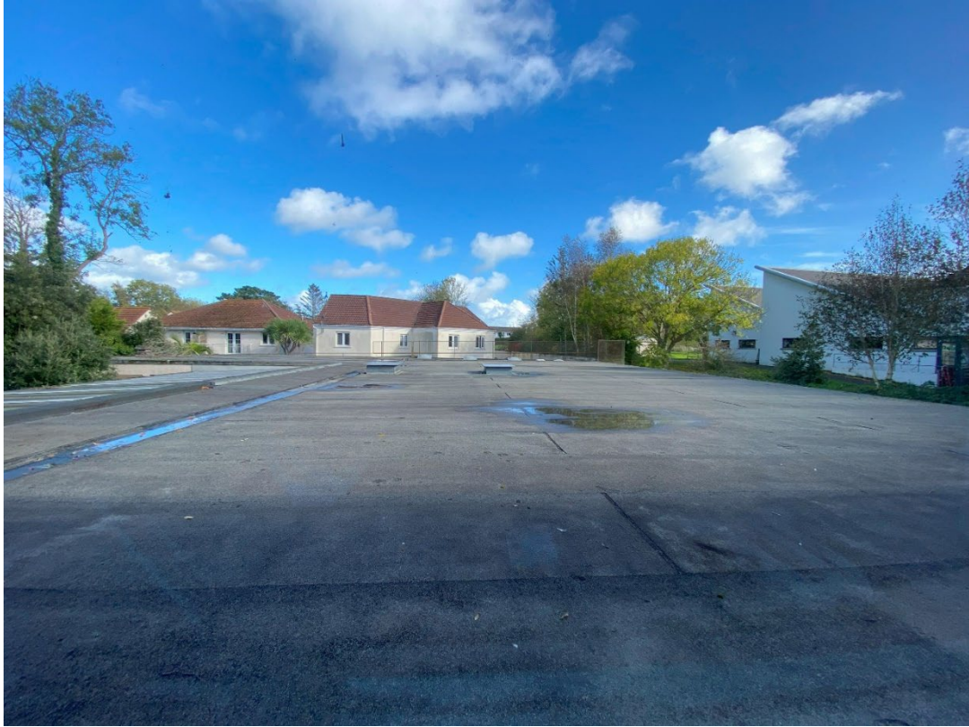
School of Art – mineral flat roof covering over first floor is aged with signs of wear and ponding
