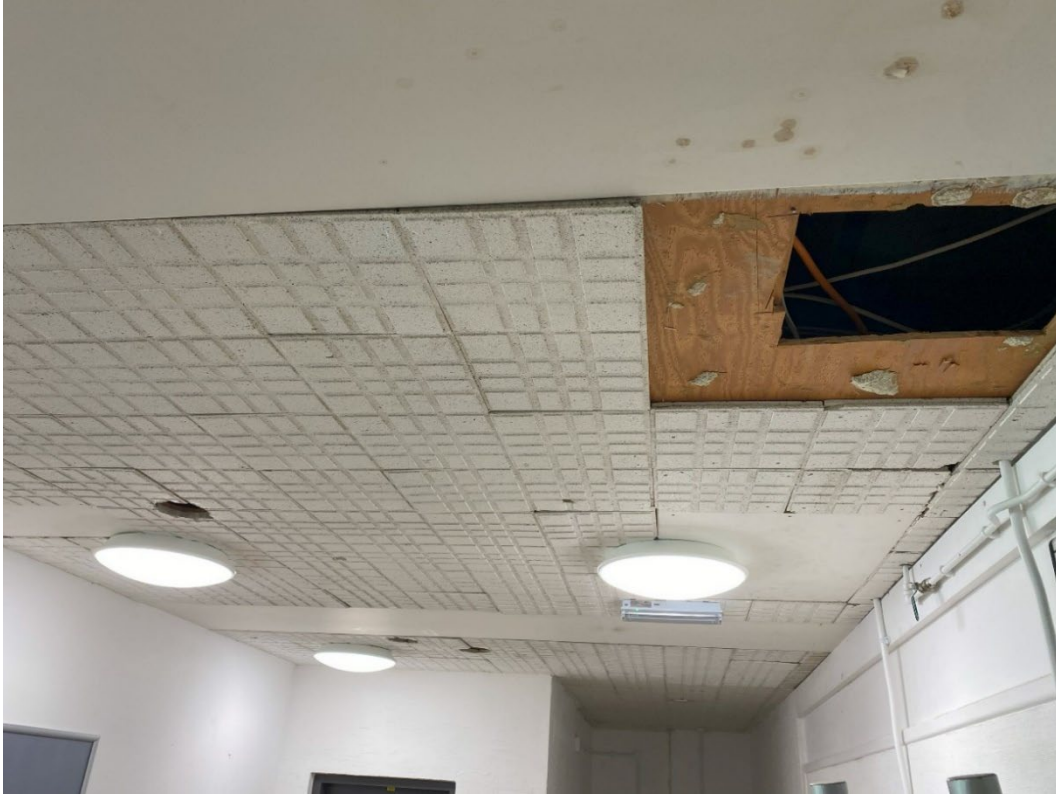
Sport and Media – condition of ceiling panels is very poor due to their age and recent water ingress.
