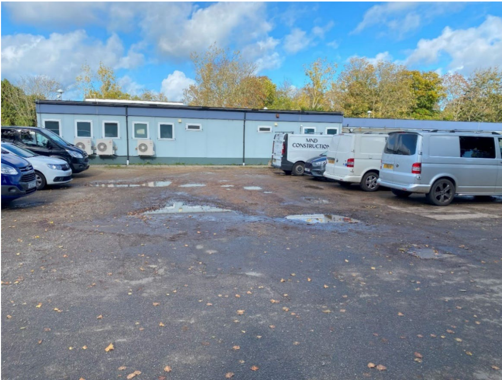
D'Hautree Car Park – surface has significantly deteriorated leaving a number of potholes presenting a hazard for pedestrians and vehicles
