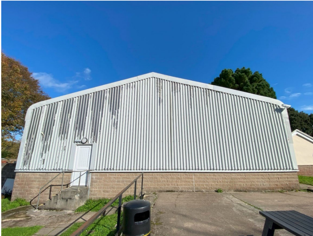
Nash Building – steel portal frame – significant corrosion to sections of the framework and supports. Worst affected areas seen to front elevation as a result of water ingress to window surround.
