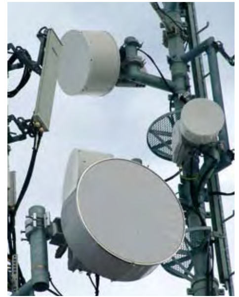
These directional antennae on the Jakobshorn (canton of Grisons) link mobile phone base stations and switching centres over relatively short distances.
