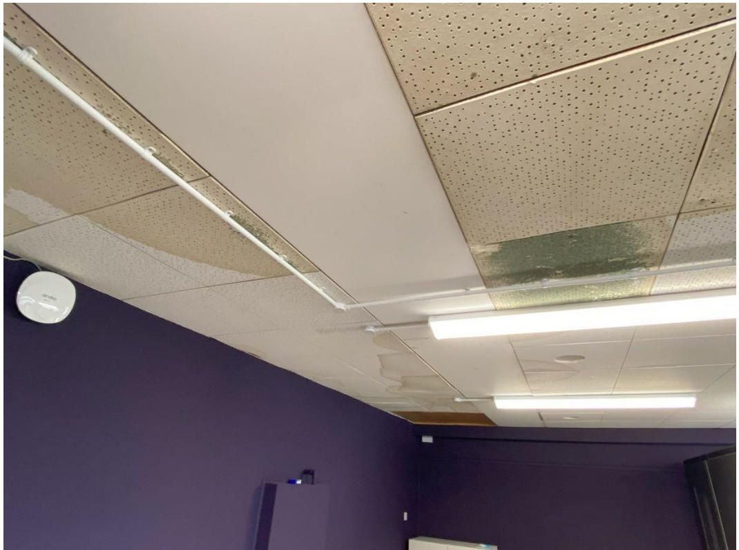
Sport and Media – Room 004 – mould and water staining from recent water ingress presents health and safety hazards
