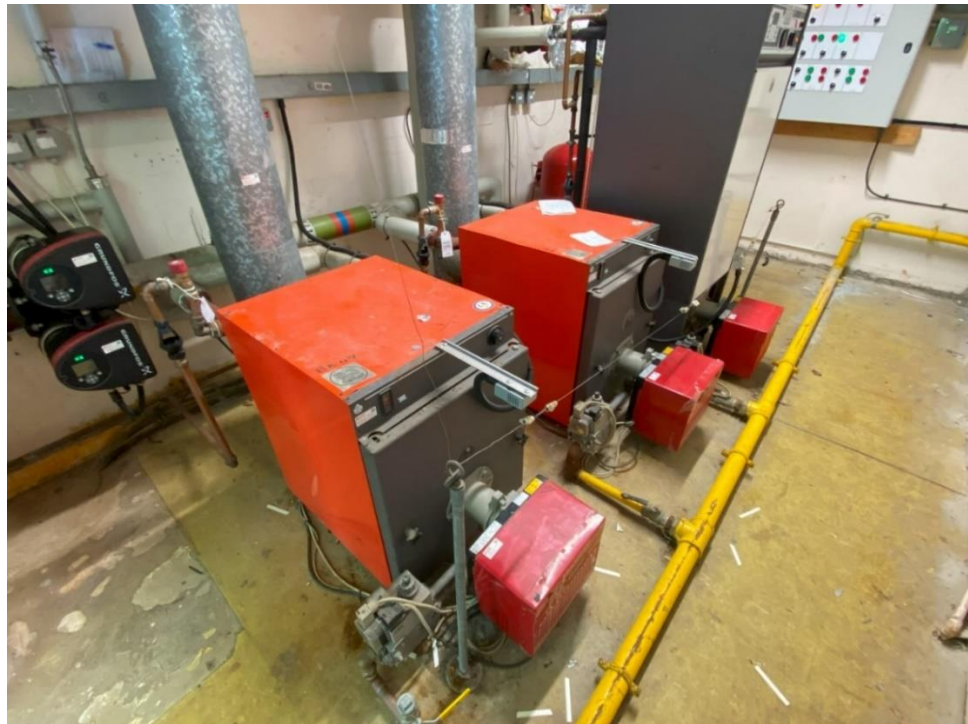
School of Art – Ground floor – two gas fired boilers and external burners require replacement being beyond their economic life
