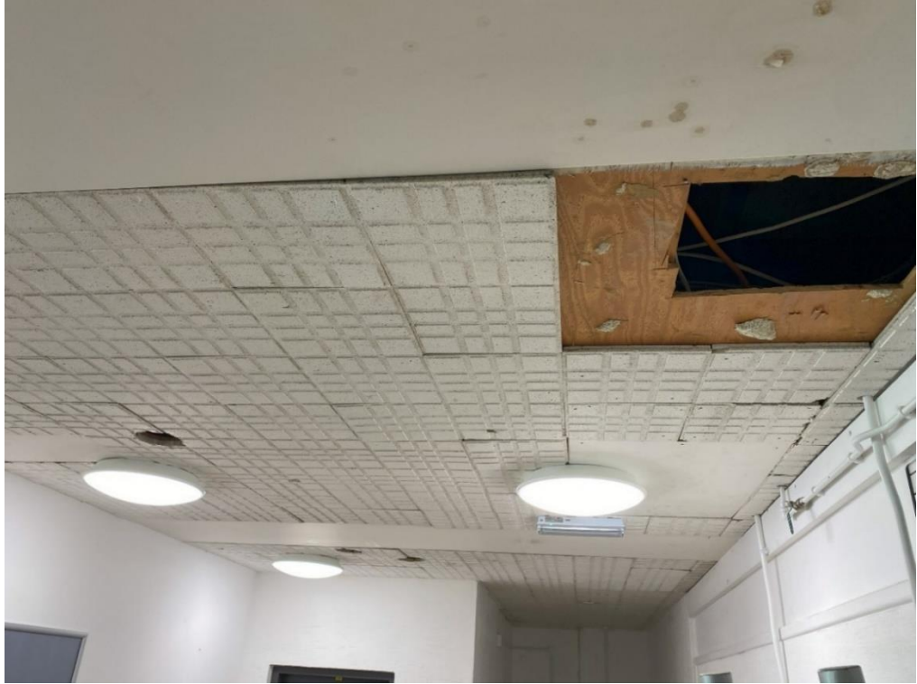
Sport and Media – condition of ceiling panels is very poor due to their age and recent water ingress.
