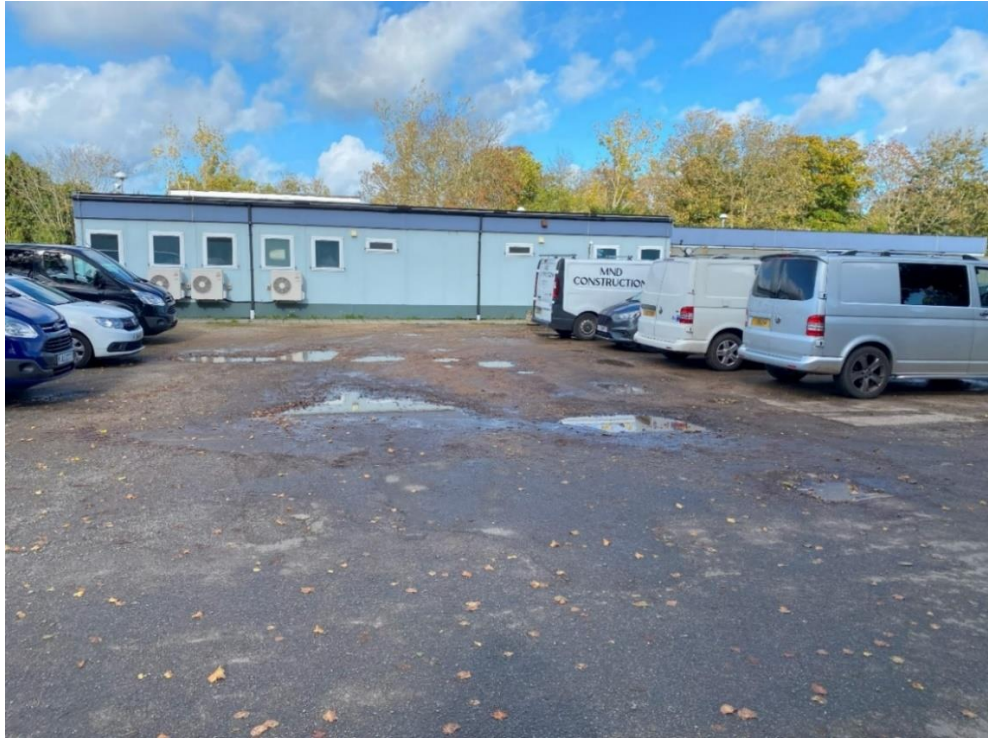
D'Hautree Car Park – surface has significantly deteriorated leaving a number of potholes presenting a hazard for pedestrians and vehicles
