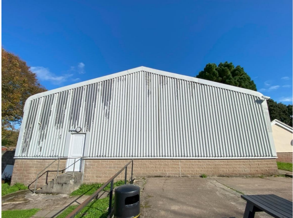
Nash Building – steel portal frame – significant corrosion to sections of the framework and supports. Worst affected areas seen to front elevation as a result of water ingress to window surround.
