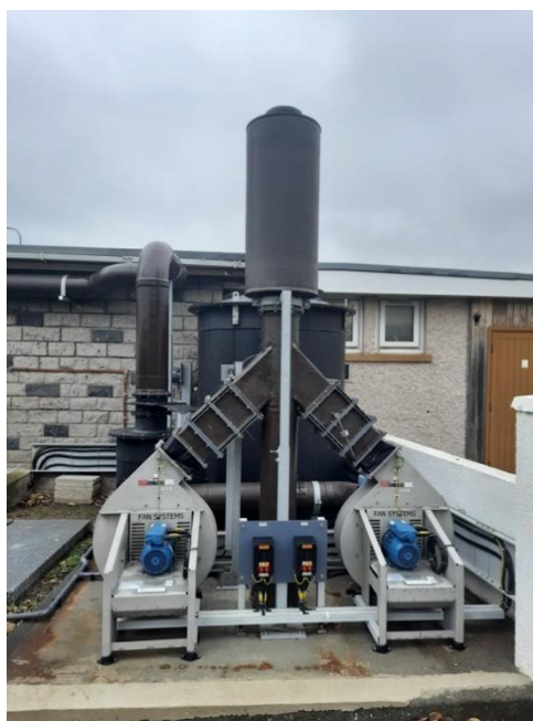
Photo B1.8.2 : Le Hocq odour control system
