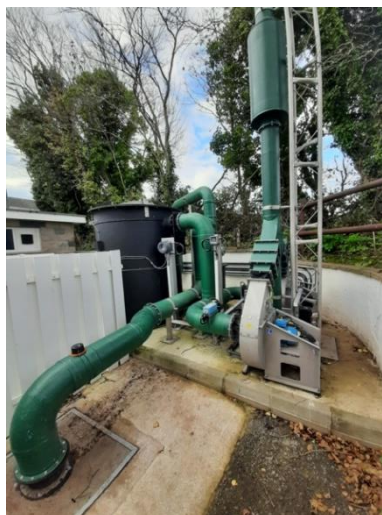
Photo B1.9.2 : Pontac Odour Control equipment
