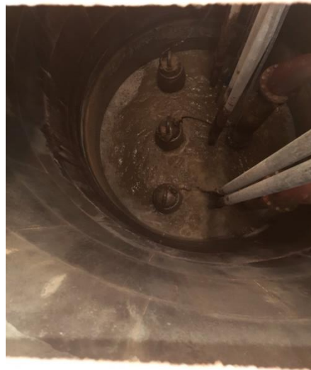
Photo B1.8.4 : Le Hocq main pump wet well
