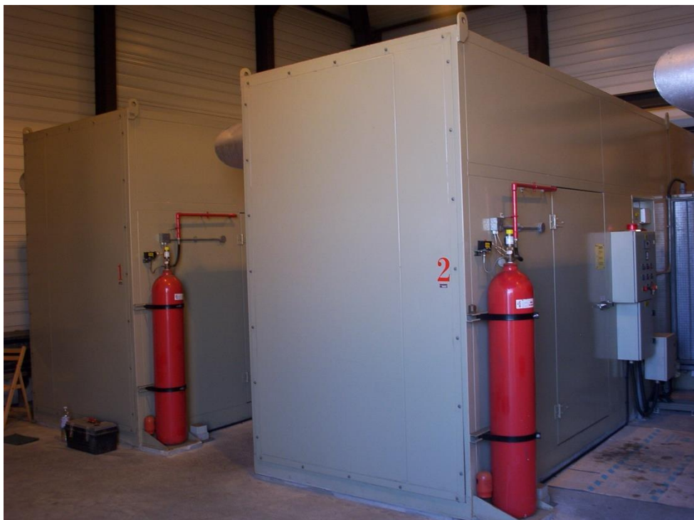
Photo J3.3 : West of Albert Pump 1 and 2 Engines
