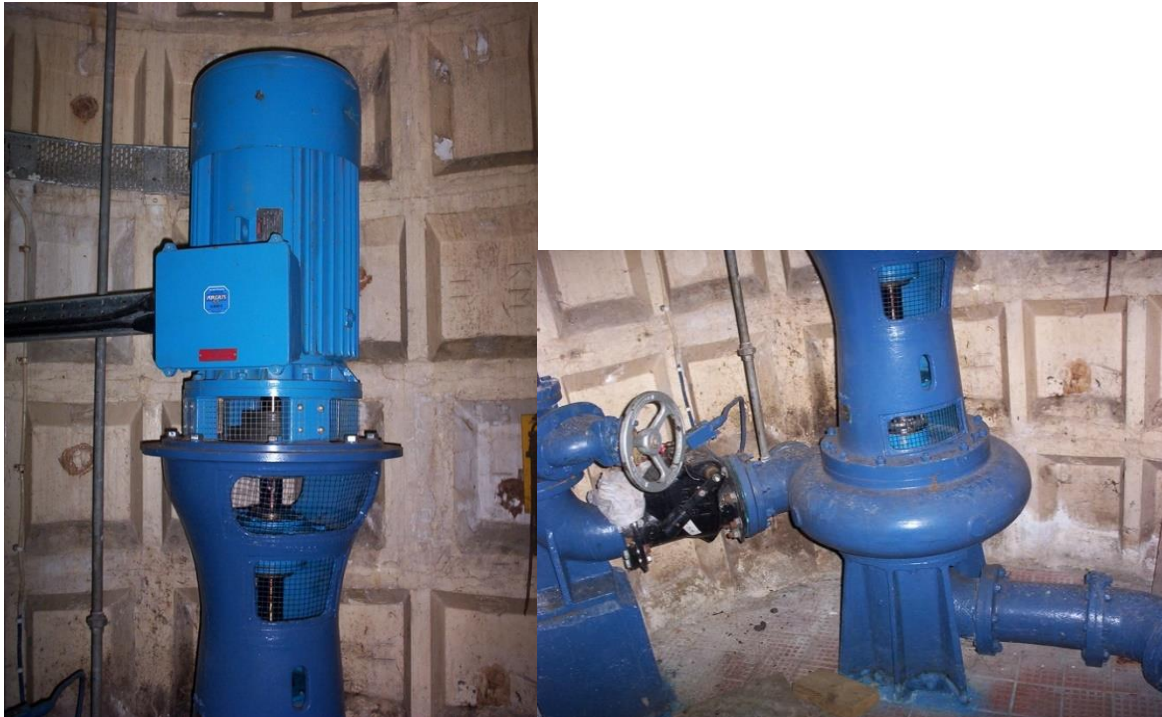
Photo B1.7.2 : Dry well mounted pumps
