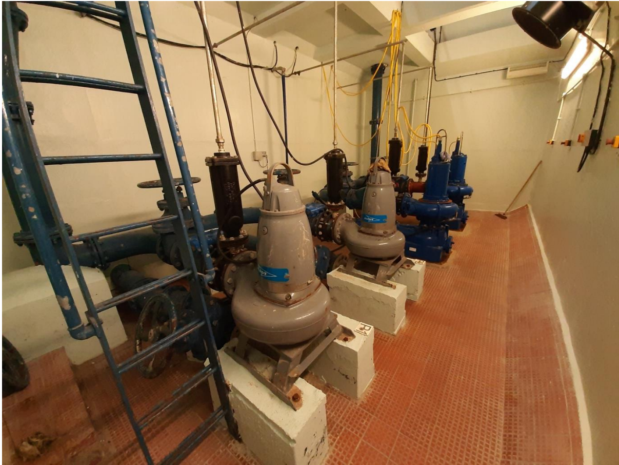
Photo B1.3.2 : Beaumont pumping station dry well configuration
