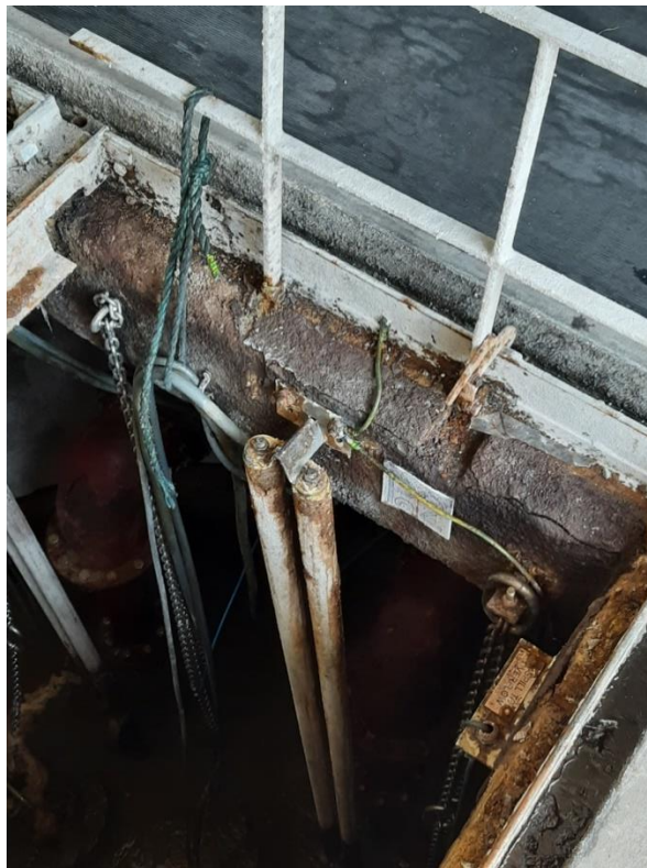
Photo E1 : Atlantic Pumping Station signs of Hydrogen Sulphite Attack
