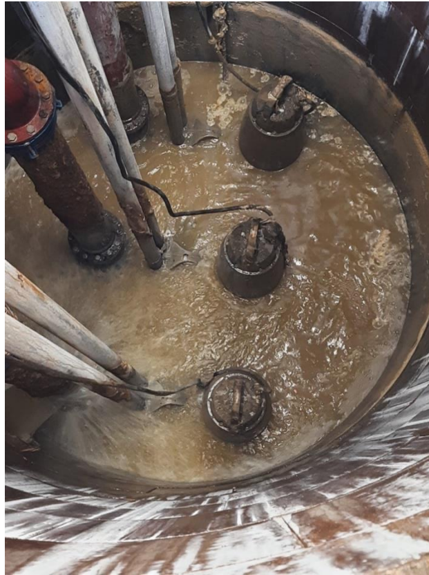
Photo B1.9.3 : Pontac main pumping station wet well
