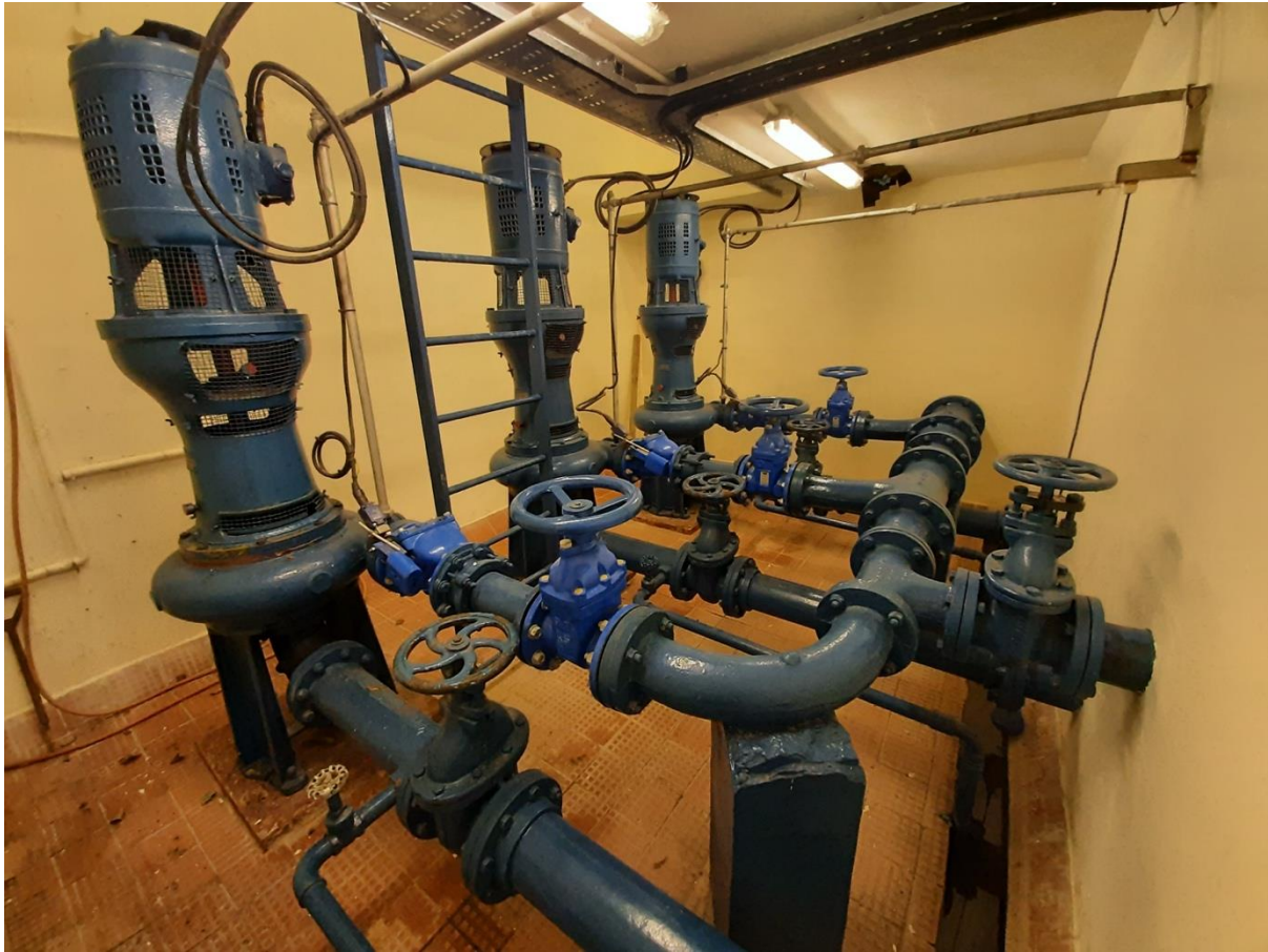
Photo B1.6.3 : Route Orange Dry well pump configuration
