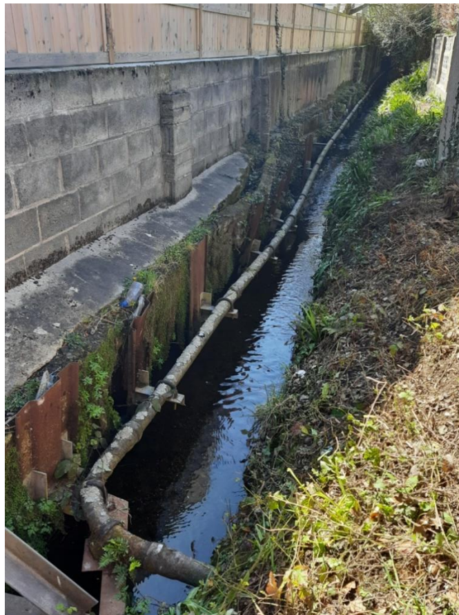
Photo E2 : Fountain Lane rising main
