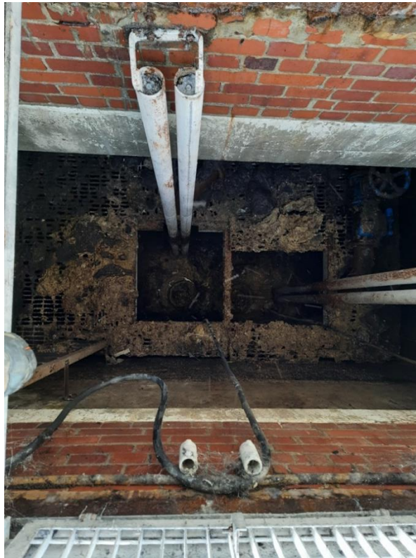
Photo B1.4.3 : St Brelades no 1 wet well pump installation
