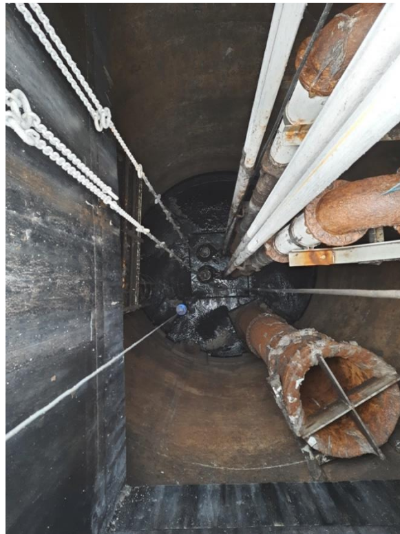
Photo B1.5.4 : Maupertuis Overflow sump pumps
