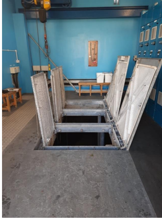
Photo B1.5.3 : Maupertuis Sewage pumping station wet well
