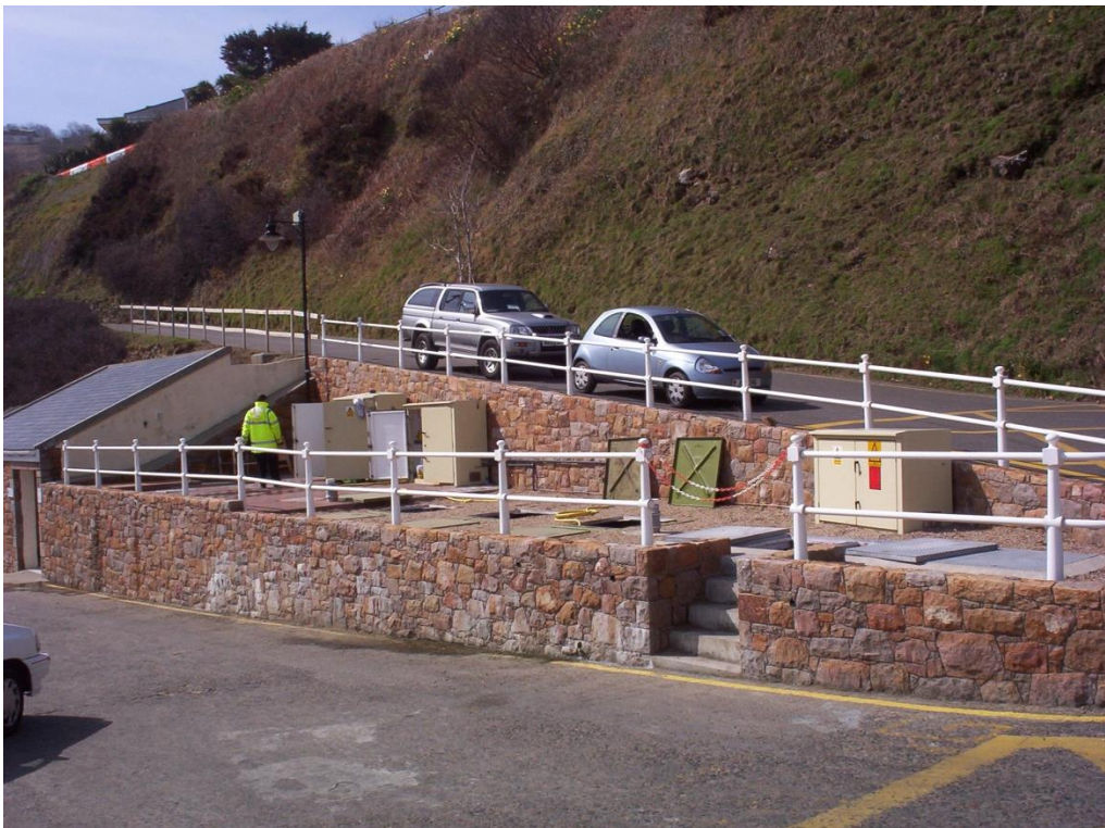
Photo J1.1 : Bonne Nuit treatment plant
