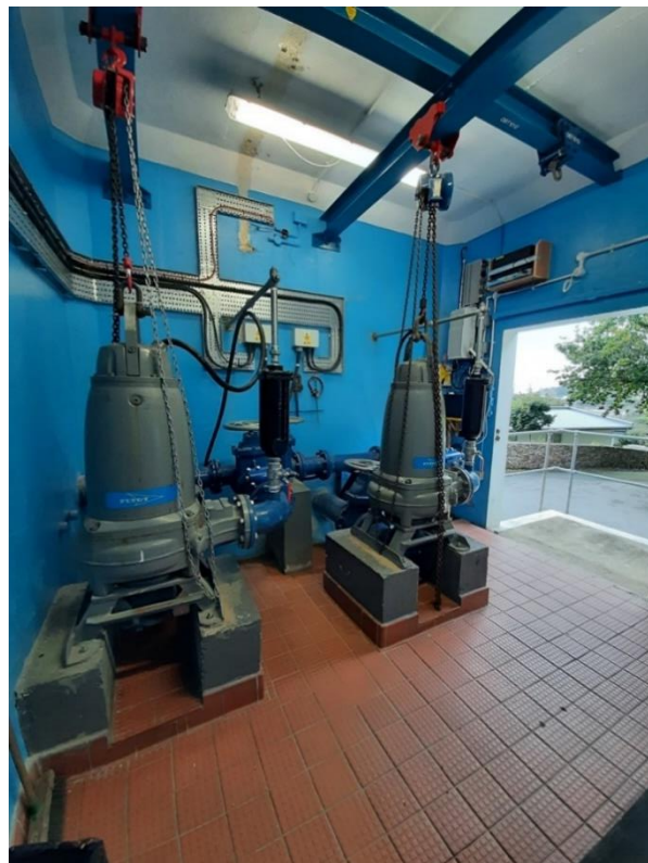
Photo B1.4.4 : St Brelades no 2 dry well configuration
