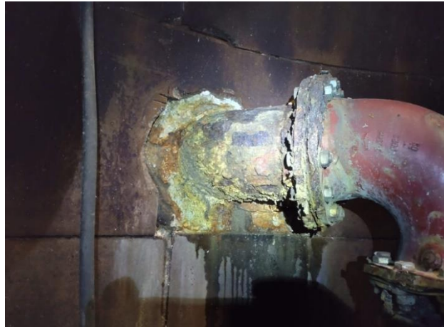
Photo B1.8.5 : Le Hocq interface with the rising main
