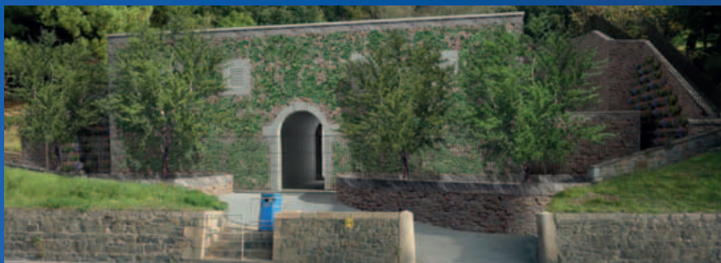
Work has started on St. Helier West primary substation which is expected to be in service in 2016
