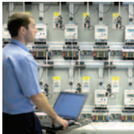
Richard Marriott, Meter Technician tests the latest in smart meter technology prior to their installation in a new residential development
