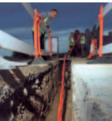
Jason Baines, Network Services Engineer supervises the ongoing reinforcement of our underground HV transmission network
