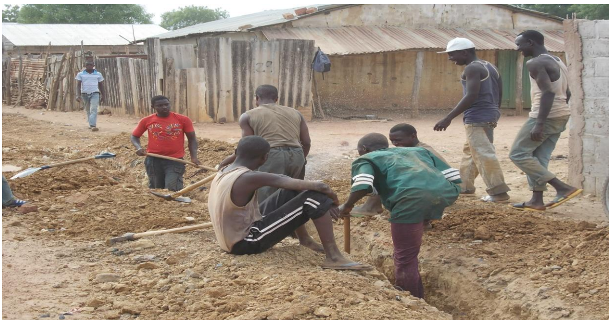
The Community at Janjanbureh, Gambia, preparing the trench for JAPs water and sanitation project.
