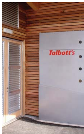
Biomass boiler, Kingsmead School. Source: Cheshire CC
