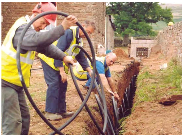
GSHP has reduced CO 2 emissions from Gamblesby village hall by 75%. Source: CLAREN
