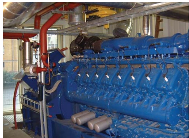
CHP plant, Woking. Source: Woking Borough Council
