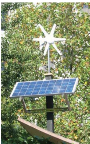
Small-scale 500W wind turbine with a PV array. Source: XCO 2
