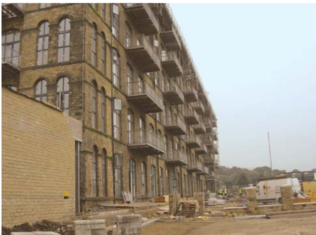
Energy and water systems for a converted mill managed using an ESCo. Source: ESD Ltd
