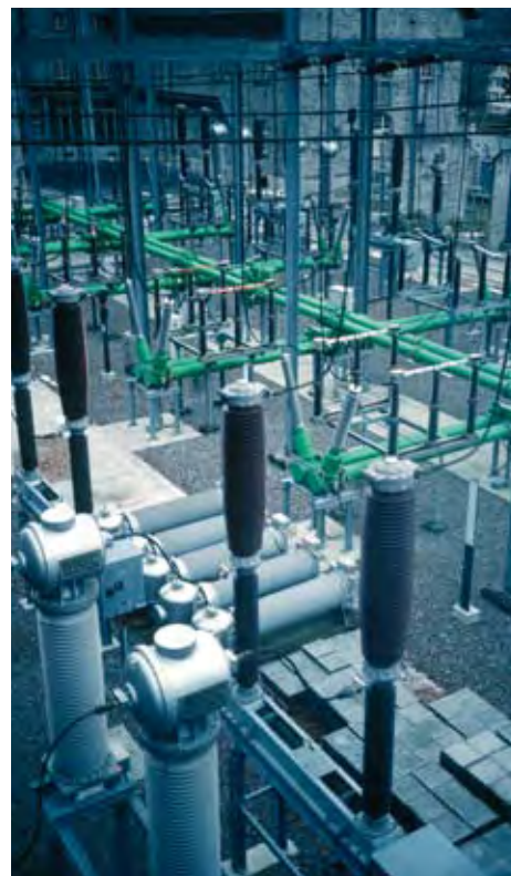
In addition to high-voltage power lines, sub-stations, too, produce relatively intensive magnetic fields within their fenced-in area.
