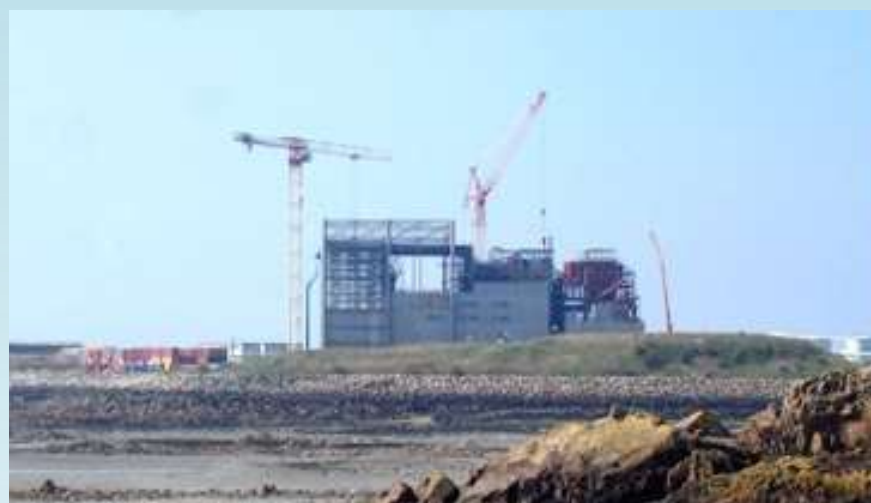
The incinerator under construction; the early ash mounds are on the right, rusting containers containing asbestos on the left Photo: SOS Jersey, 10 April 2010
