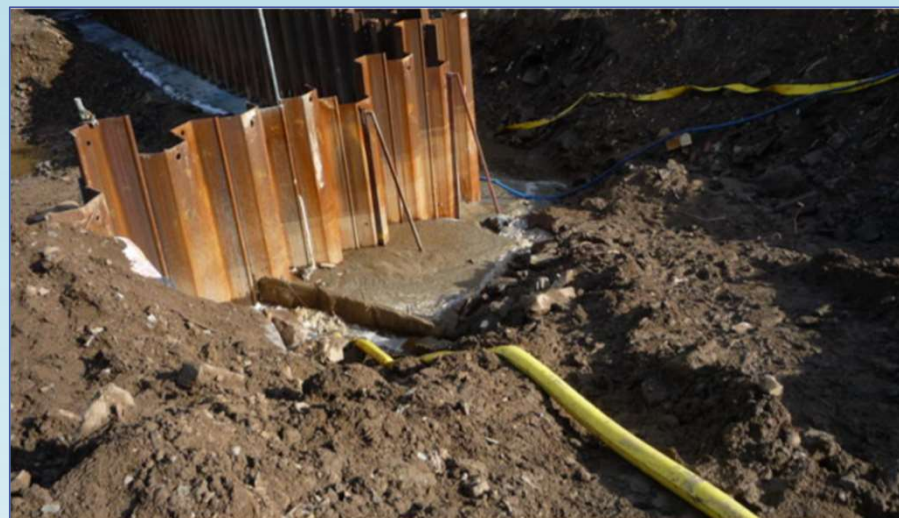
Above: Contractors illegally pumped toxic leachate into the Ramsar area of La Collette via the cooling culvert belonging to JEC (now Jersey Electricity) Photo: SOS Jersey, 2009
