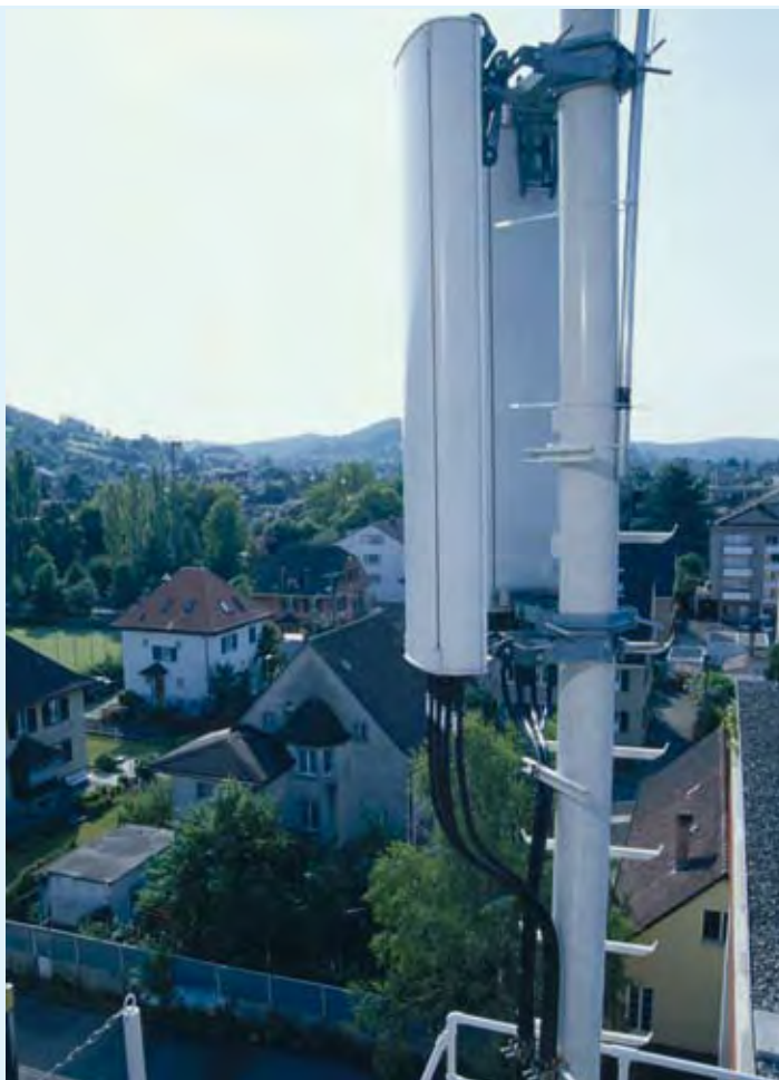
The antennae installed at base stations establish contact with mobile phones within their range.
