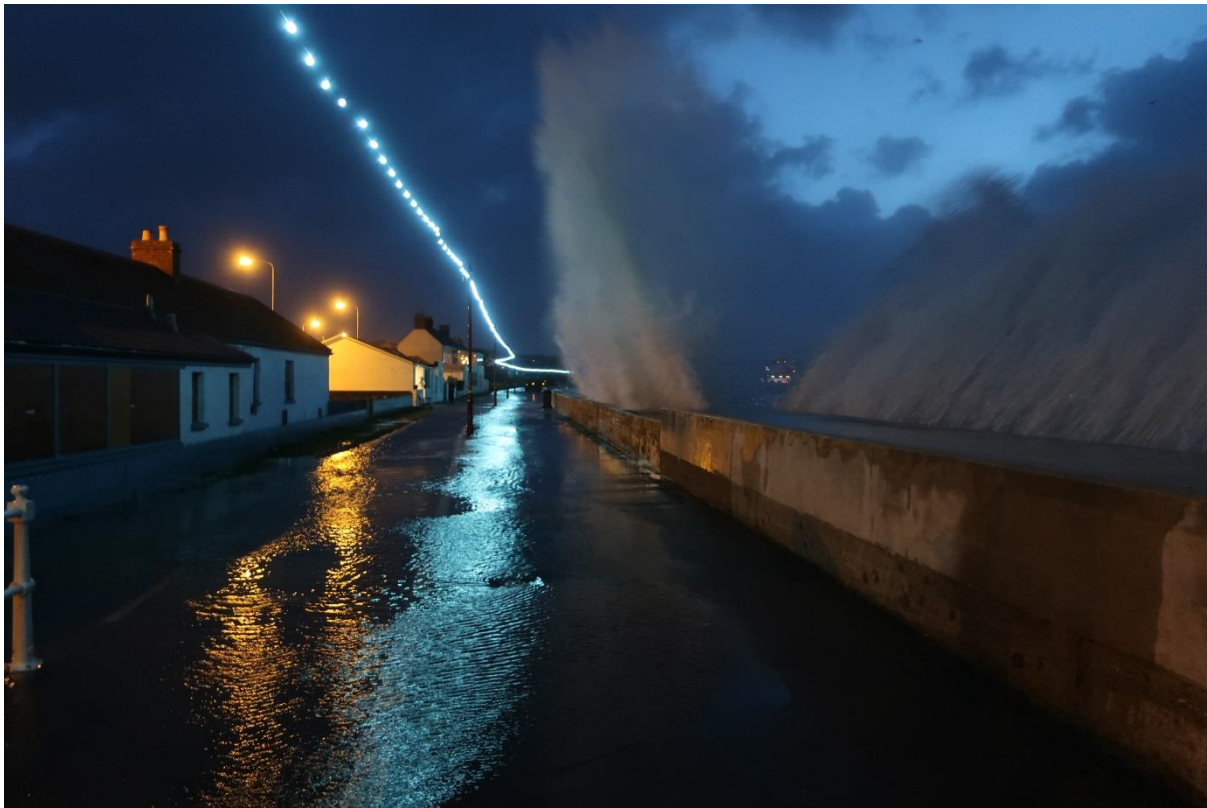
Figure 4-13: Recurve wall design at Gunsite, St Aubin's Bay (CMU 1.5)
