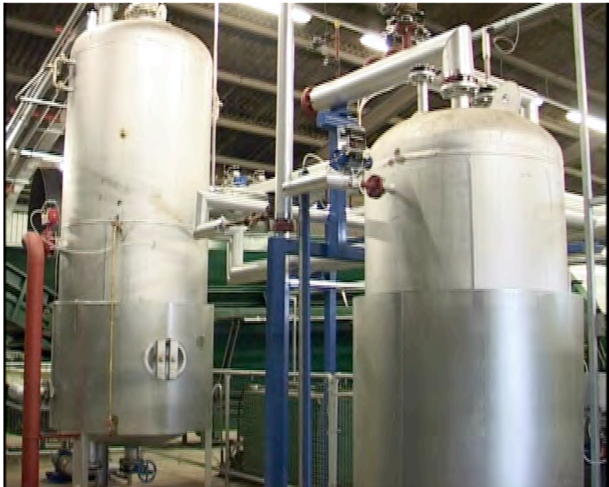
Steam condensate vessels
