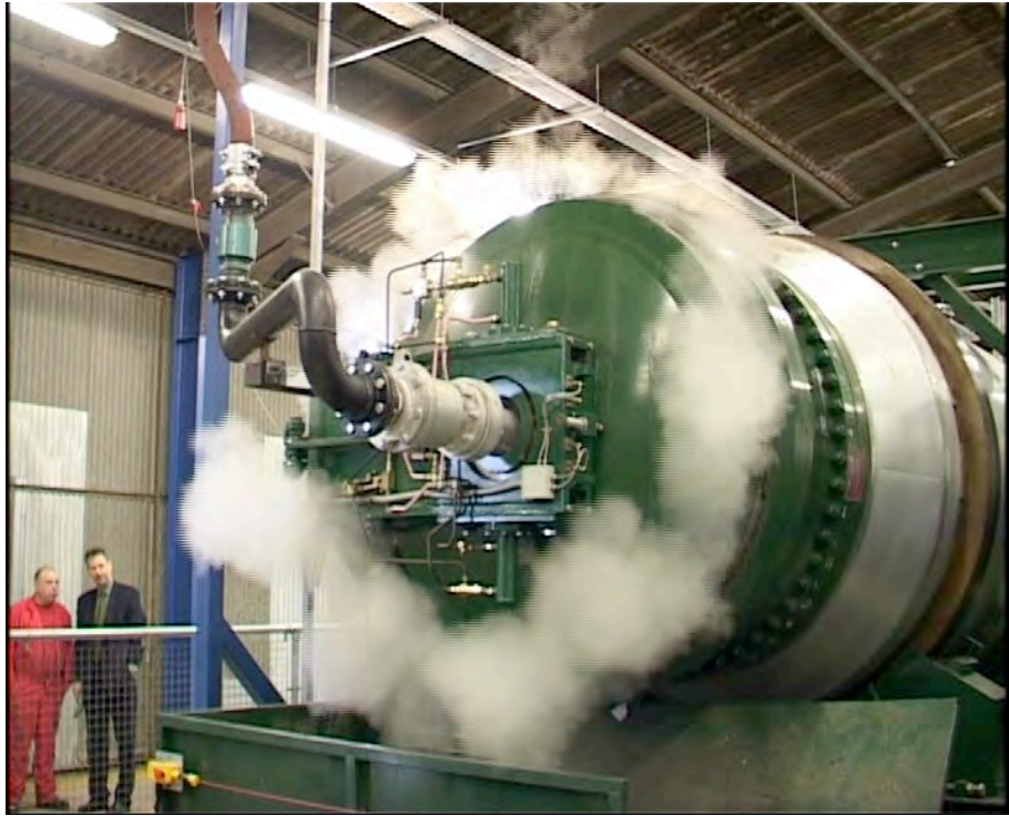
Autoclave opening after pre-treatment process
