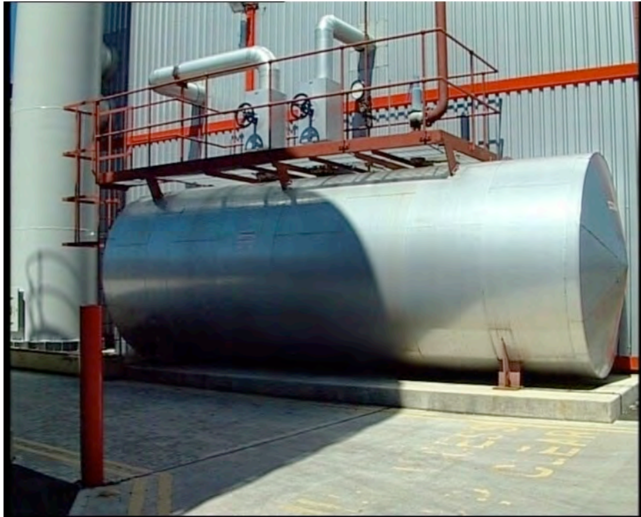
Steam Accumulation / Storage vessel
