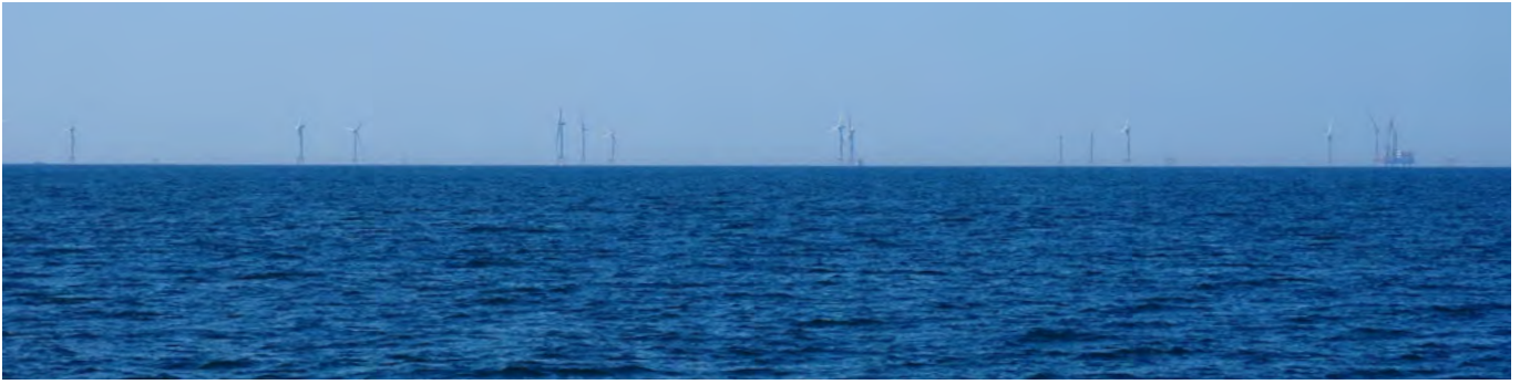
The St Brieuc windfarm under construction in French waters (as seen from Jersey waters, south-west of Les Minquiers).
