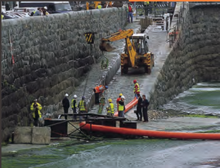
The powerline finally arrives in Guernsey's Havelet Bay and the CIEG is complete.
