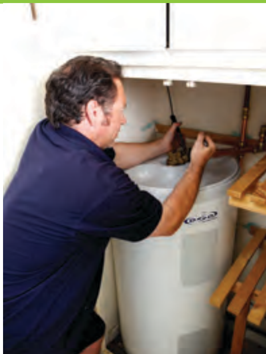
Ian Campbell, JEBS Plumbing and Heating Engineer, fits one of the highly insulated, efficient hot water cylinders at Les Cinq Chenes as part of the States Housing Switch Project.
