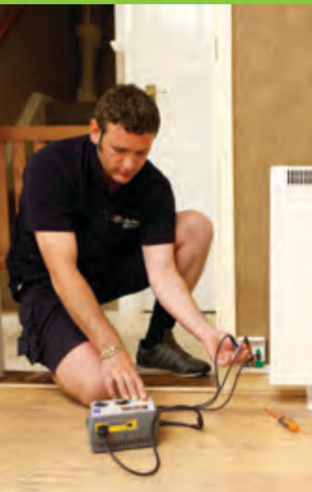
Chris Young, JEBS Electrician, tests a new installation of storage heating at Les Cinq Chenes as part of the States Housing Switch Project.
