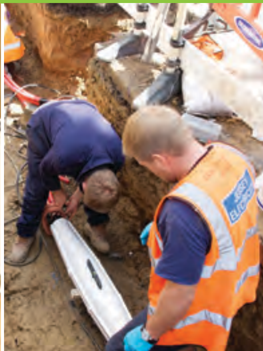
Andy Barker, High Voltage Joiner, and Robert Pike, Apprentice Joiner, connect a cable.
