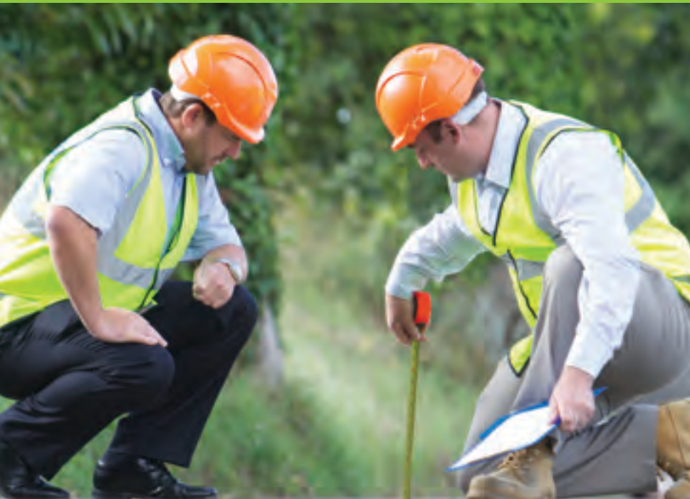
Jeremy Willis, Senior Project Engineer, and Jason Baines, Construction Engineer, survey a site for new cable laying.
