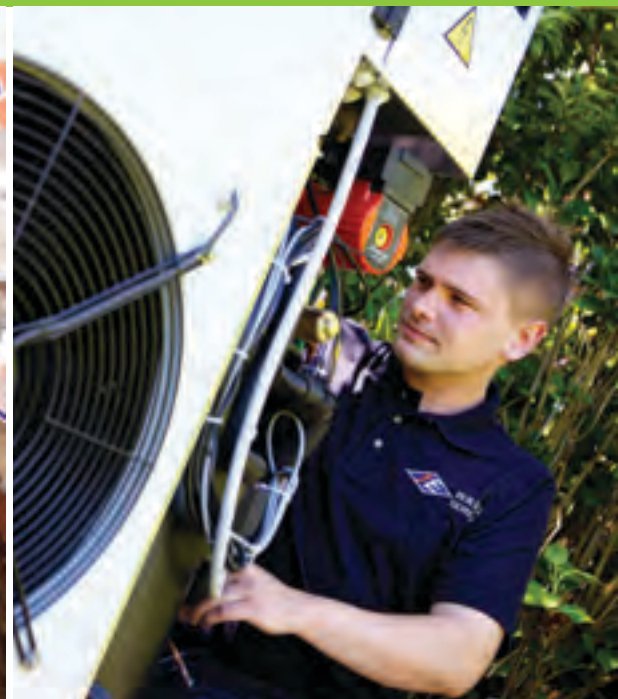
Danny Oberst, JEBS Plumbing and Heating Engineer, makes the final connections to one of the latest heat pump installations.
