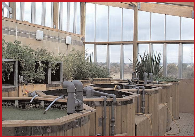
BedZED's living machine on-site sewage treatment plant
