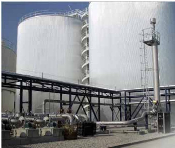
Mechanical-biological waste treatment plant for MSW and separately collected municipal biowaste (from Linde website)
