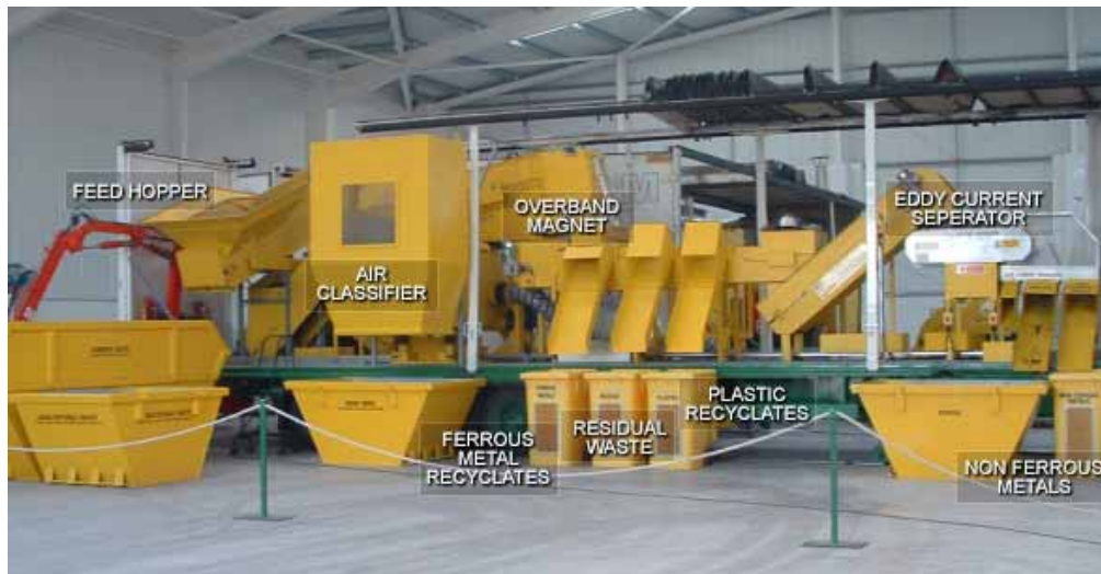
Materials Separation equipment
