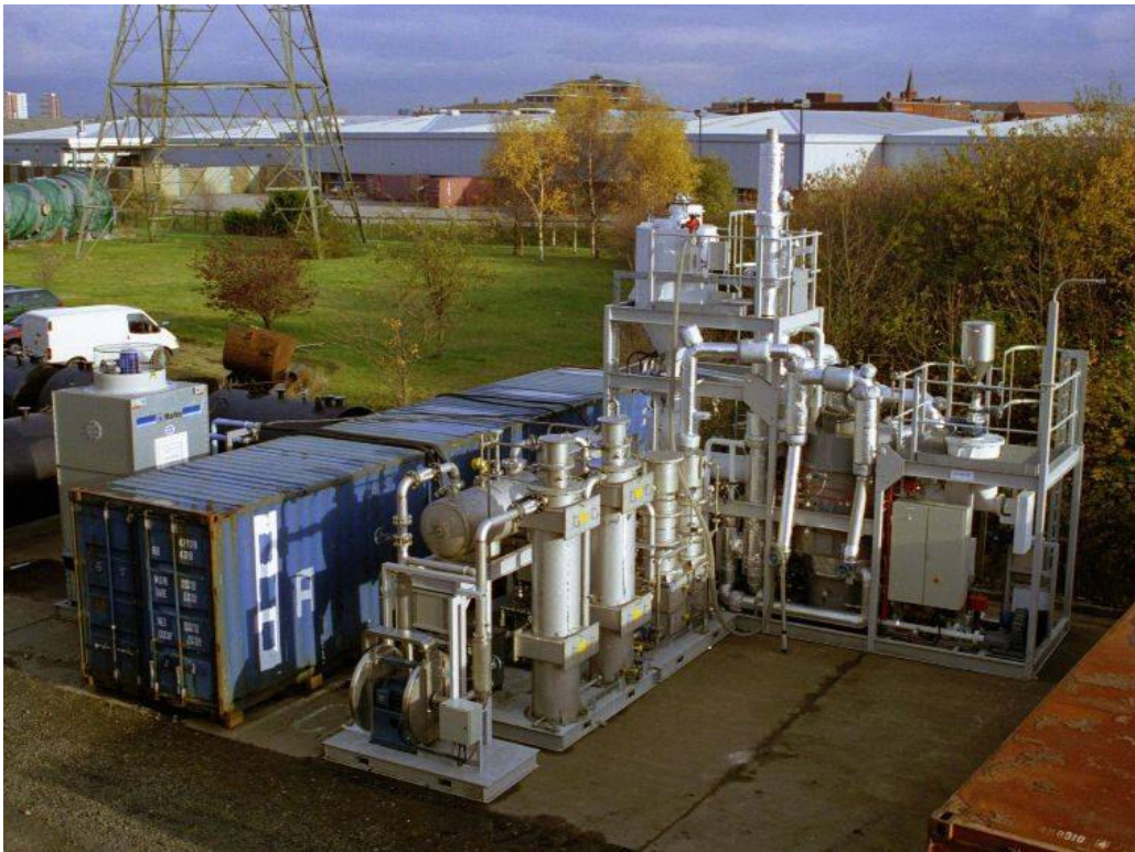
Integrated Fast Pyrolysis Plant
