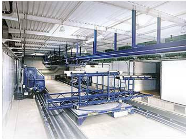
MBT plant, Borken Germany (from Linde website)
