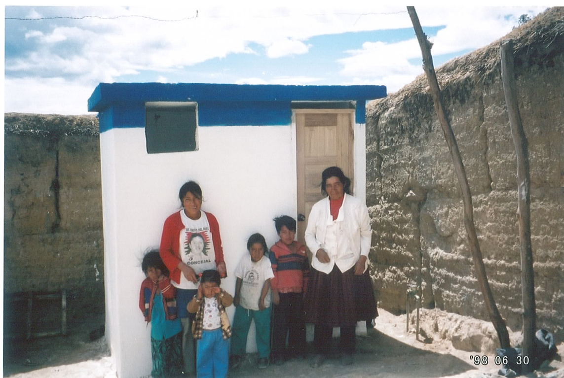
A family stands outside their newly installed toilet and washing facilities. Ecuador Plan UK
