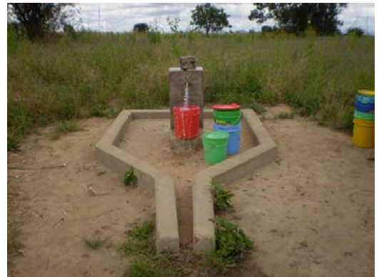
Picture of a constructed water point
